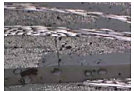
Cross section of crack formation in composite
